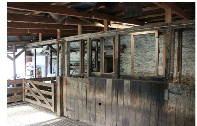
This portion of the wall appears to be the earlier extent of the original woolshed. Propose to retain this wall located between the circulation spine and the dining area
