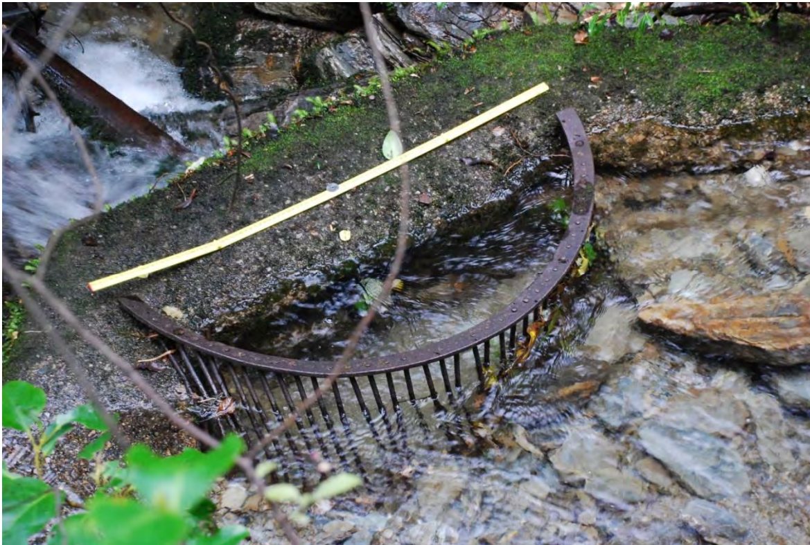
Photo 2 The half-round iron grill protecting the mouth of the supply pipe at the weir (with yellow 1000mm rule).
