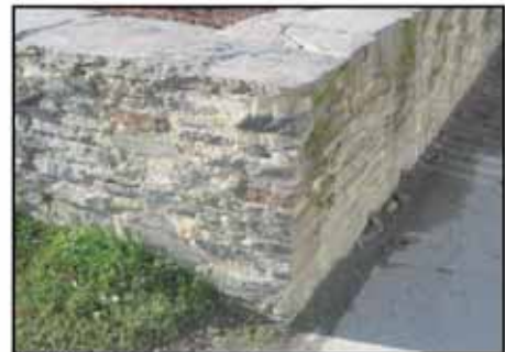
Mortared walls. Stick to local stone, i.e. do not use Alexandra stone.
