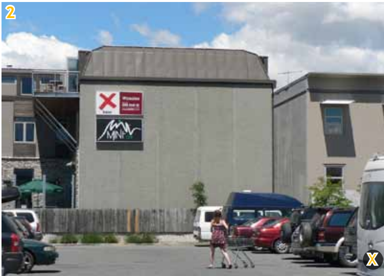
Bland blank wall exposed to public area
